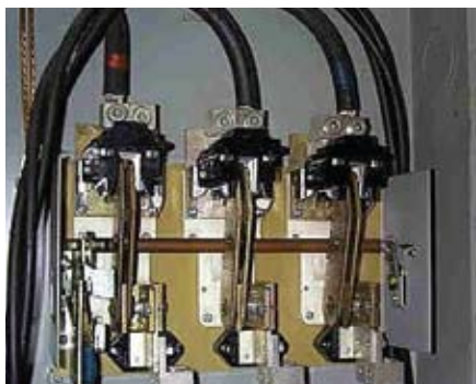
Thermal photograph reveals a fault on one phase of a three phase disconnect switch.
