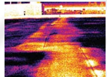
Thermal photograph showing heat loss through a roof membrane.
